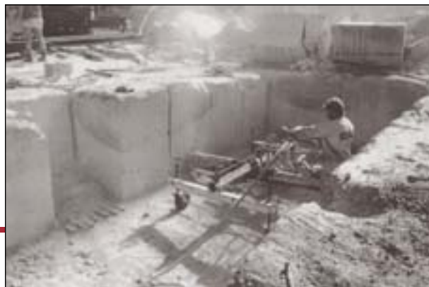
Sandstone being cut at the cathedral quarry, Helidon. Stone is now being taken in horizontal cuts rather than this older style of verticle sections.
