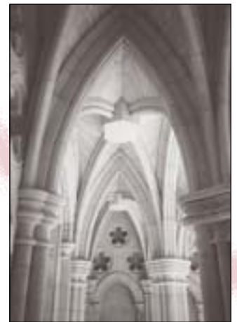
1997 This stone-vaulted ceiling in the Lower Gallery is just one sample of the ancient craft which forms every ceiling space in St John's, as specified by original architect John Pearson
