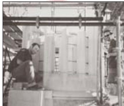
2001 L to R, James Turvey & Brendon Rackett building the South Turret of the West End.
