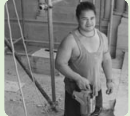
Cathedral builder Joe Elisaia with jackhammer preparing space for the foundation of the major weight-bearing column of the northern tower.
